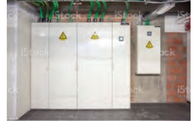
Figure 9: An electrical distribution board.
